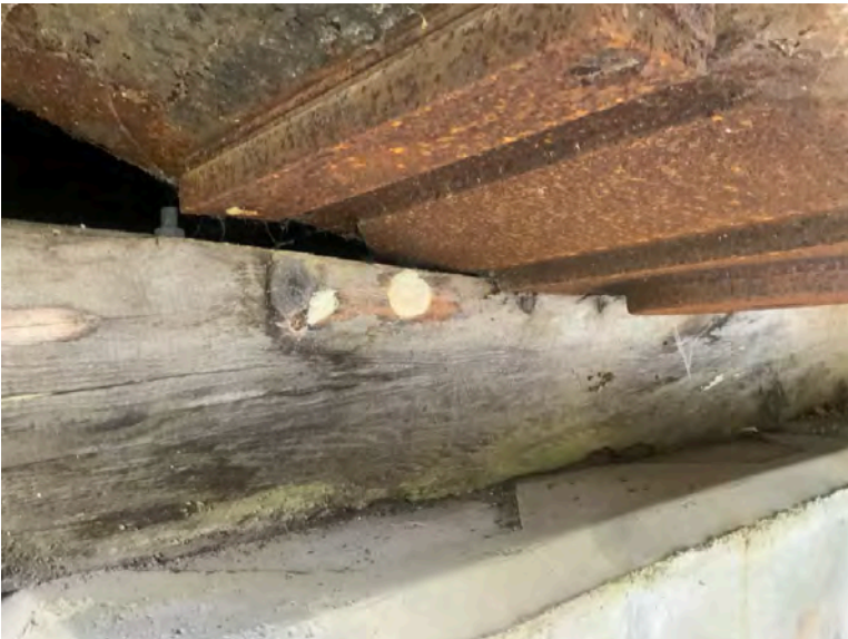
Sills showing age and crushing
